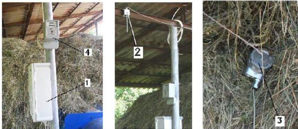
Fig. 3. Electrical command and control system: 1 – control panel; 2 – sensor for measuring atmospheric air temperature and humidity; 3 – sensor for measuring the temperature in the feed layer; 4 – electric meter
